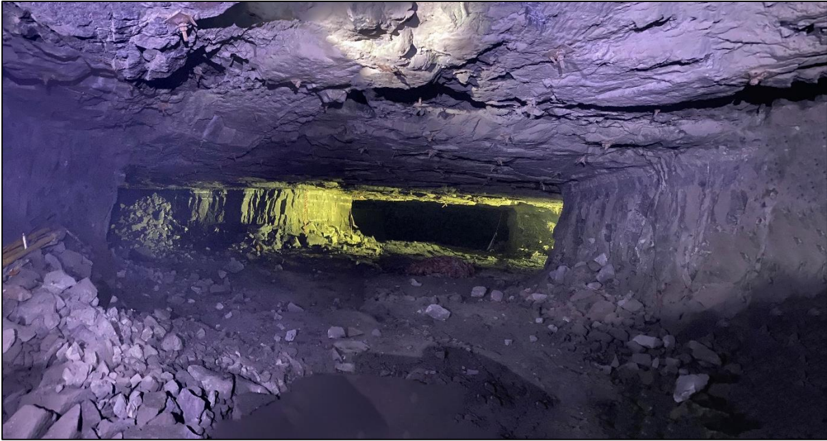
Figure 6: General condition of pillars in the Eastern sections visited
