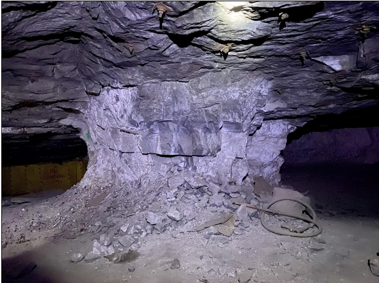
Figure 10: Deteriorating pillar along well-defined horizontal contacts.
