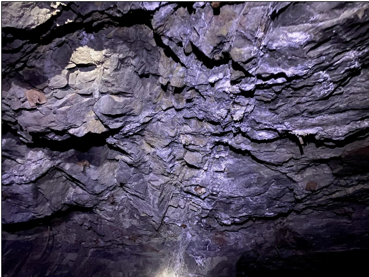
Figure 8: Typical hanging wall conditions associated with a flatter joint set resulting in rough hanging wall conditions.
